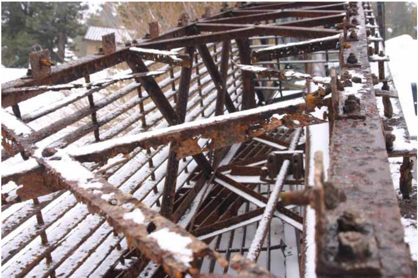
Figure 8. Silver Lake outlet tower removed during the 2008 emergency repair - Notice all of the missing sections of structural bracing leaving no bracing for the lower vertical third of the tower.
