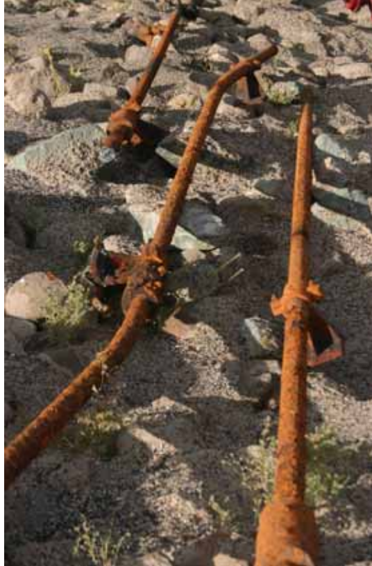
Figure 7. Section of 70 foot long Caples outlet valve stem after removal during 2008 emergency repair (notice permanent deformation).
